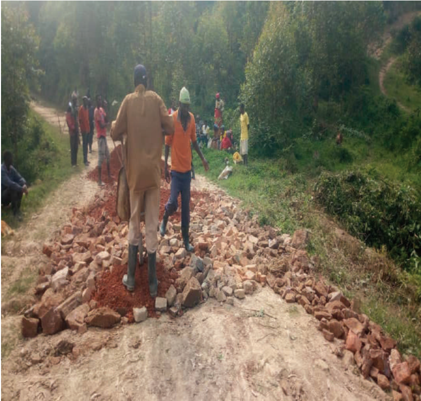
Photo 2 Men participating in rehabilitating the bridge at Nyakahita Village -Muyumbu parish -Kyanamira Subcounty.
