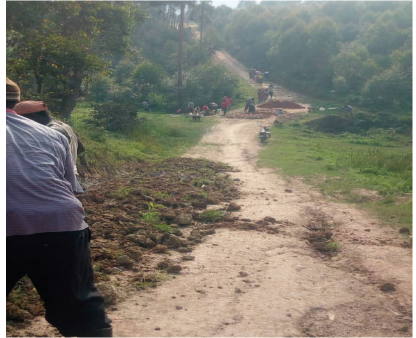
Photo: 3 Women Participating by carrying rock debris during rehabilitation of the bridge at Nyakahita Village-Kyanamira Subcounty-Kabale District.
