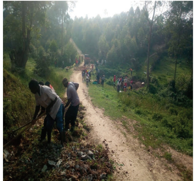
Photo: 1 Community Members clearing the road at and Rehabilitate bridge Nyakahita Village at Muyumbu Parish -Kyanamira- Kabale District.
